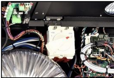
03.01 Selector inside EB
