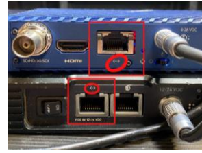
3, Make sure ethernet is connected in these ports on Serv pro & Link
