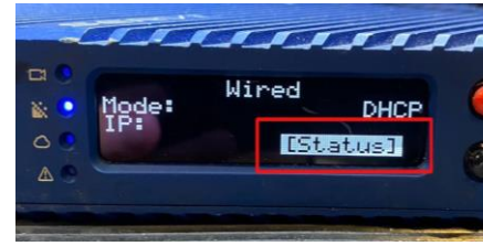
4, Check status to make sure connected properly.
